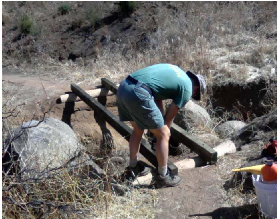
Black Mountain Open Space Park Ranger Joel Tracy is shown installing a new bridge. Photo by Senior Ranger Ed Christenson.
